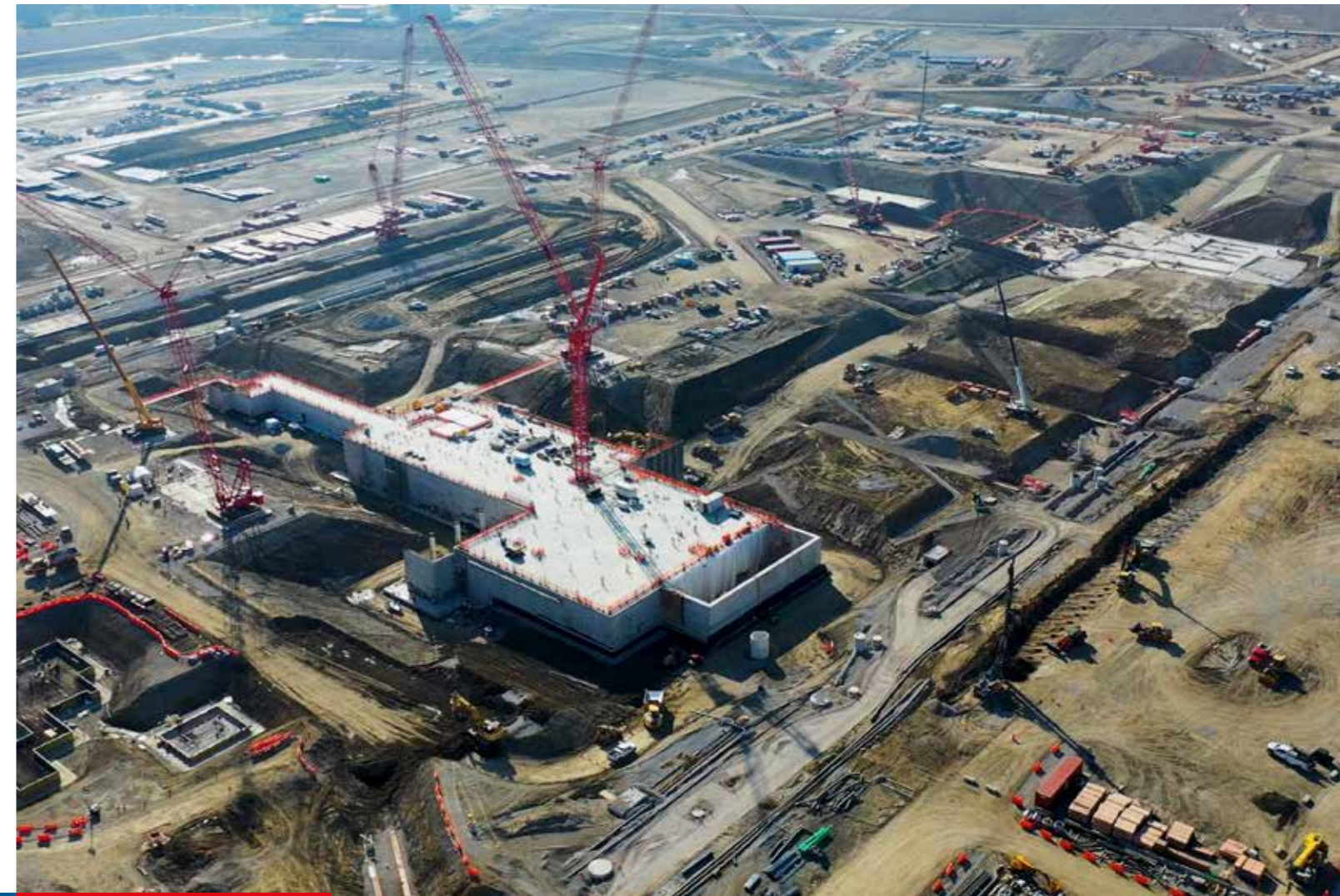
Intel Ohio One Campus, New Albany, OH, USA
